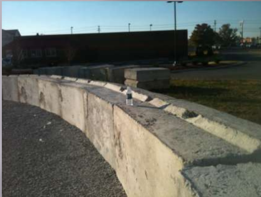
Above Ground Anchoring
